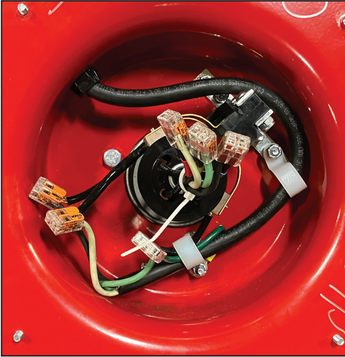
Figure 5: Final wiring of the reel
